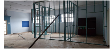
Is this a pine-framed prison? Why no, it is the CRC Offices under construction.
